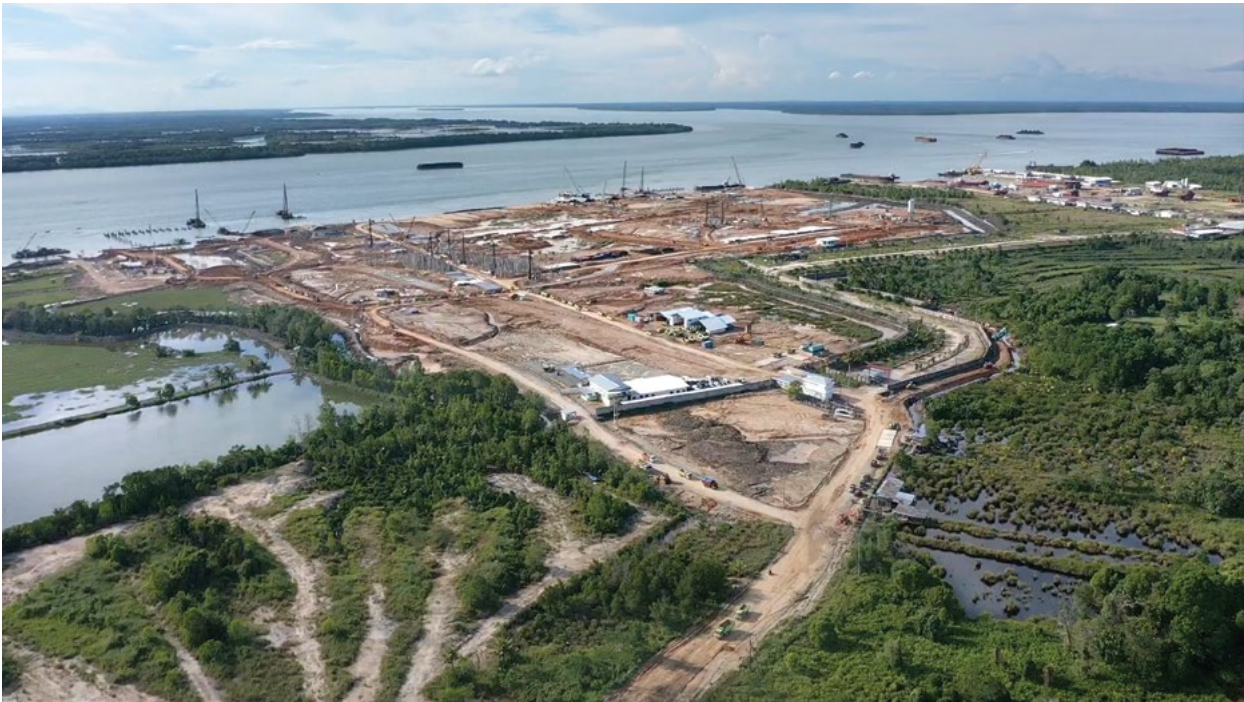
Figure 28. Construction site of PT Phoenix Resources International in Tarakan, North Kalimantan in December 2022.
